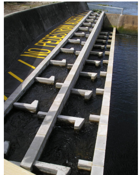
Figure 2.8.8. Vertical slot fishway installed at Mill Stream Weir 1.
