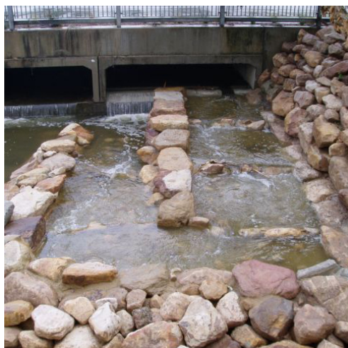
Figure 2.8.9. Partial width rock ramp fishway installed at Australia Avenue raised road culvert in Sydney Olympic Park.
