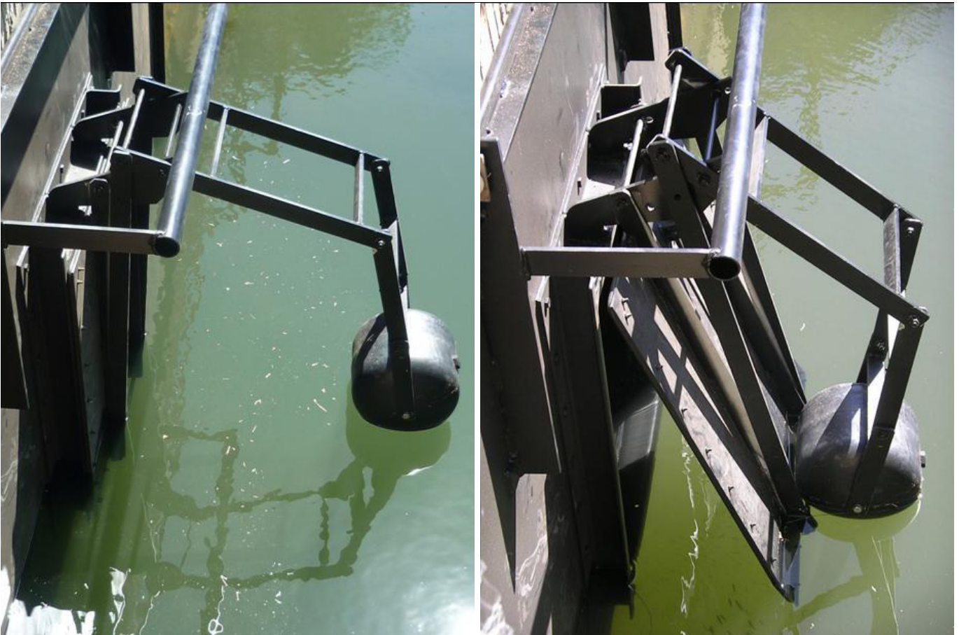
Figure 2.8.6. Auto-tidal modified floodgate in closed and open position.
