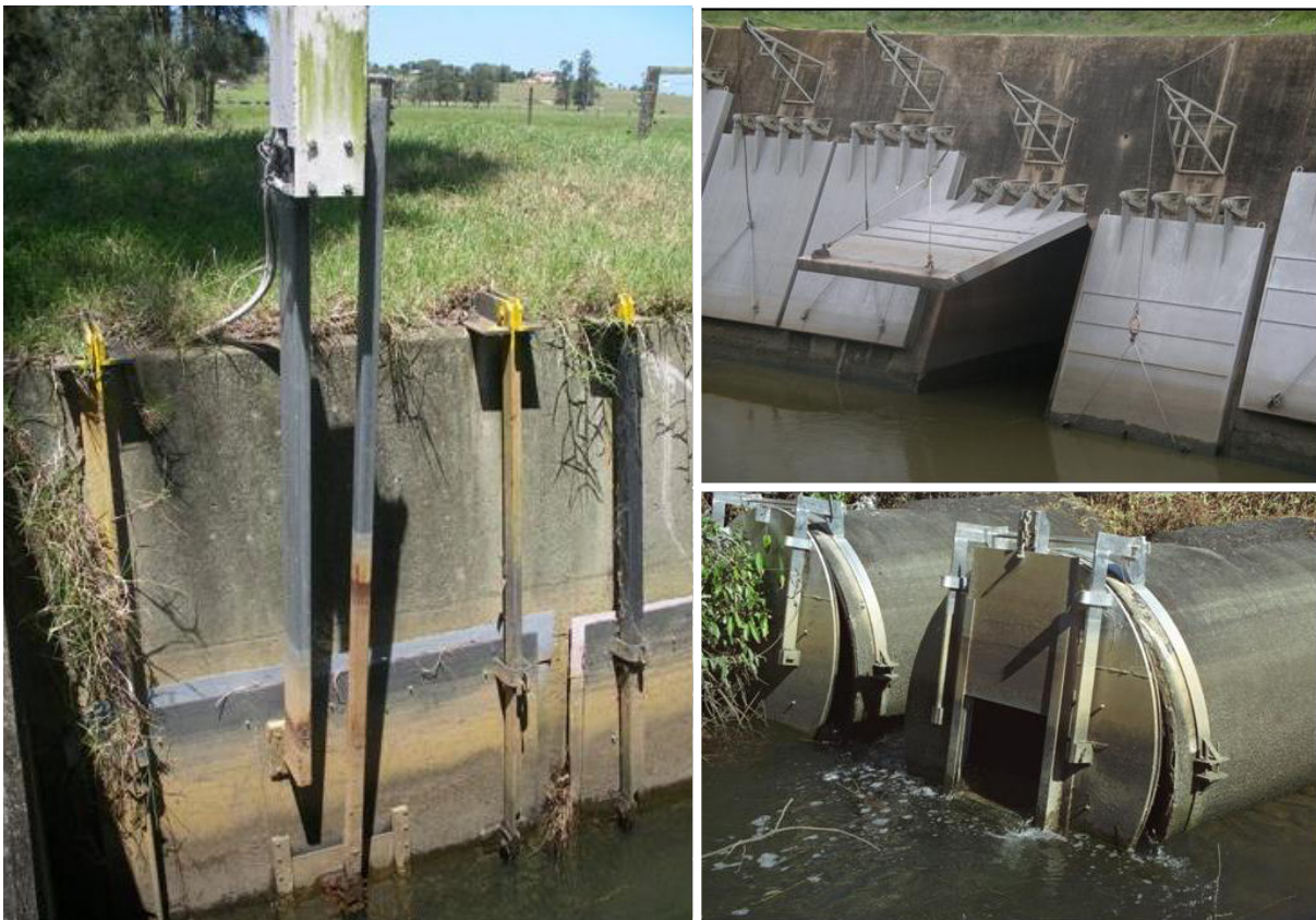
Figure 2.8.5. Smart gate (left), winch (top right) and sluice gate (bottom right).
