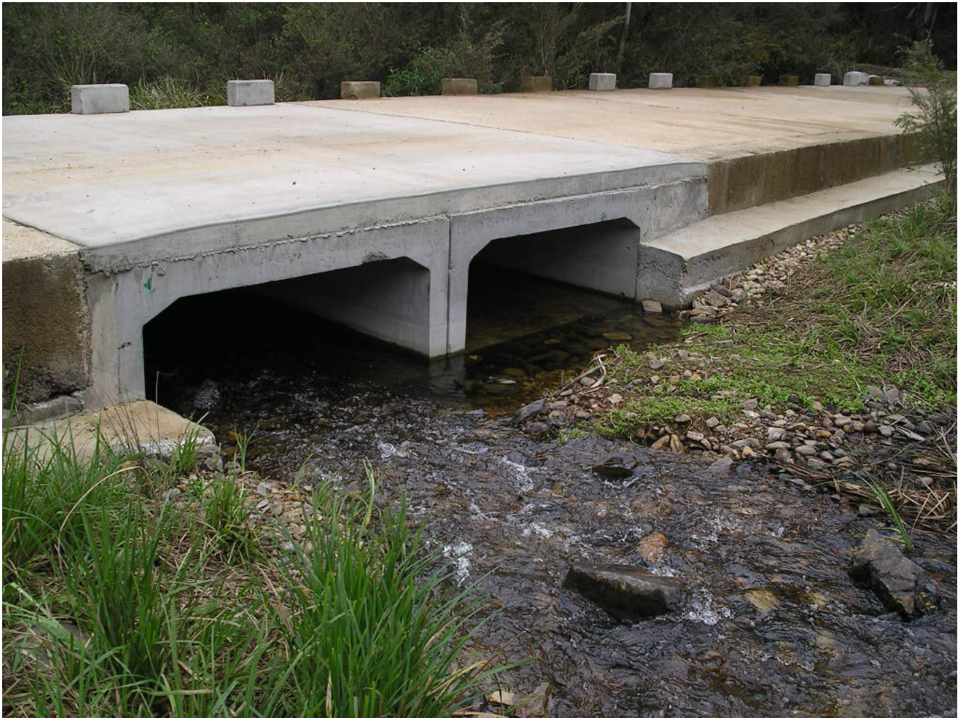
Figure 2.8.4. Road with low flow cell (left) and second cell which will take higher flows, reducing overall water velocities present.
