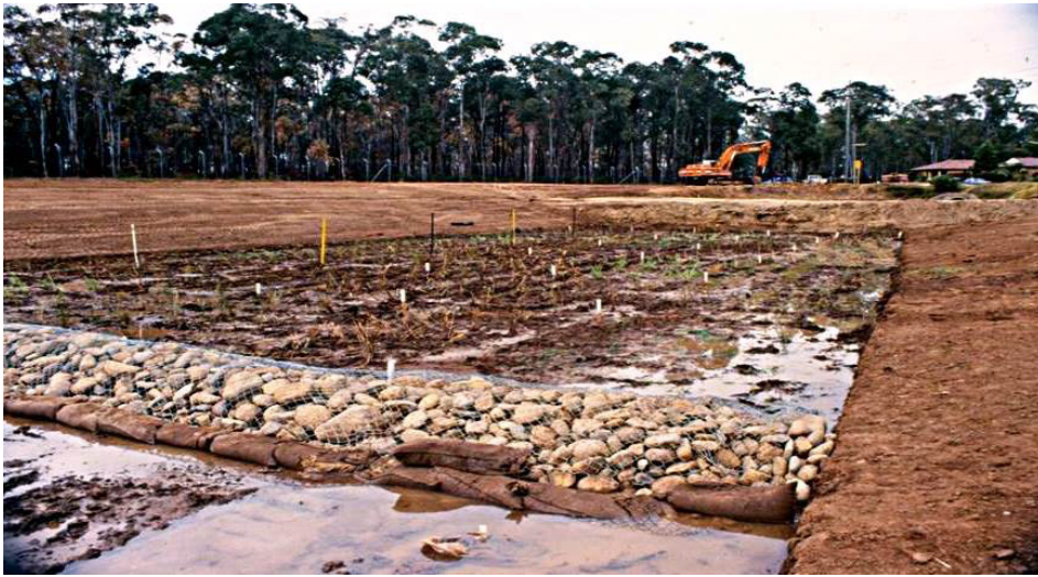
Figure 2.11.5. The marsh area at Plumpton Park, required strict level control, and isolation of each cell to control water depths during the establishment phase of the plants. Plants were placed at 2-4/ m 2 and a dense crop was achieved in 6 months. Loose rock weirs prevent short-circuiting, reduce velocity and allow access for maintenance purposes.
