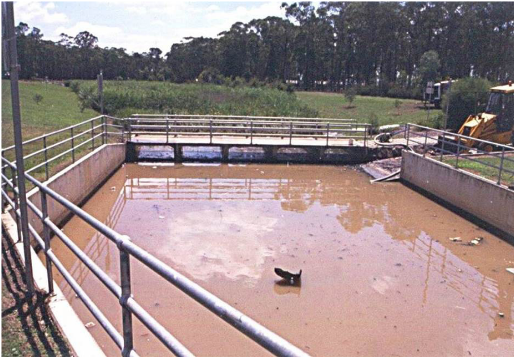
Figure 2.11.4. The GPT must be sized correctly to allow settlement of heavy pollutants and screening of floating litter. Access for maintenance is critical and draining the GPT must occur at Plumpton Park prior to the front end loader cleaning out the sediment and rubbish.
