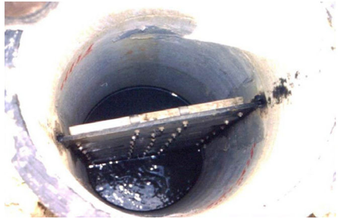
Figure 2.11.7. This Rocla Water Level Controller was used to lower the water levels in the upper cells of the Chullora Wetland to remove Carp. The ability to control the water depth in each of the wetland cells also achieved the early establishment of the aquatic plants in the Chullora Wetland Treatment System.
