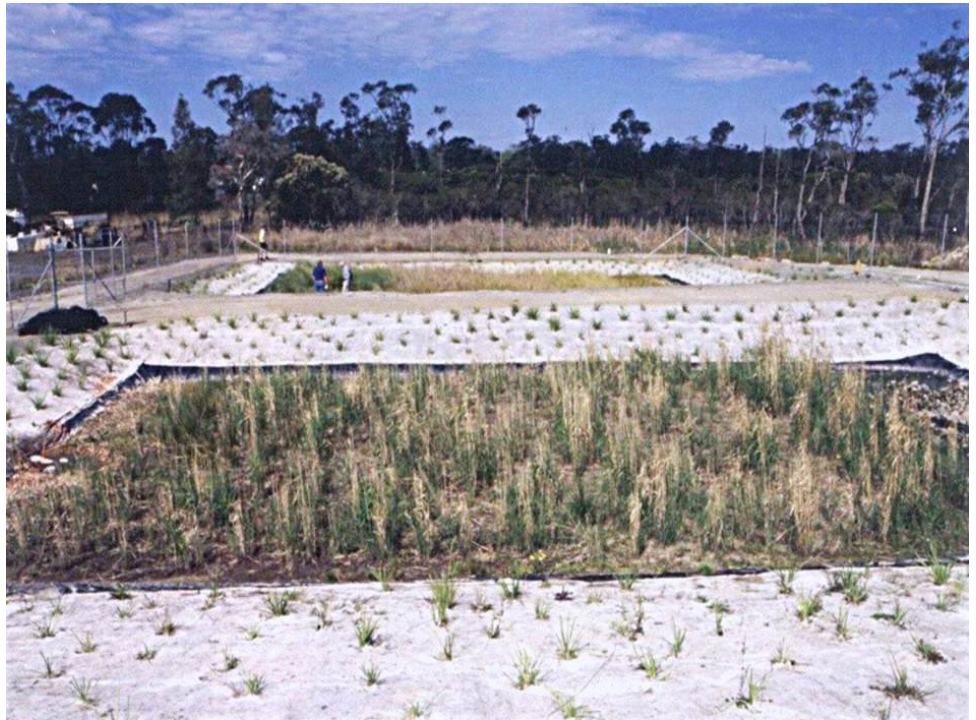
Figure 2.11.3. Runoff from a residential subdivision (Approx. 25 ha) at Blue Haven is treated with a GPT, a free water surface wetland and 2 sub-surface wetlands before discharging to a SEPP 14 estuarine wetland downstream. The sub surface wetland provides a high level of soluble nutrient and suspended solid control and reduces mosquito habitat.
